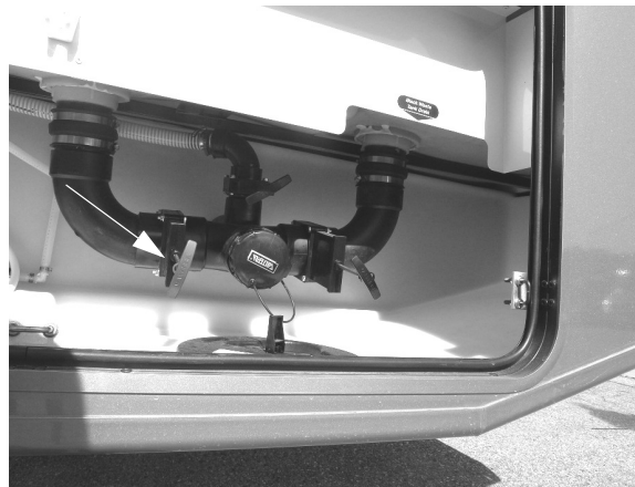
Gray Waste Tank Drain Valve (Located in water service center) -Typical View
