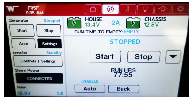
Generator Settings Screen Use this screen to customize various triggers to automatically start and stop the generator. Select the down arrow for further customizations and options. The total run hours are also displayed on this screen -Typical View
